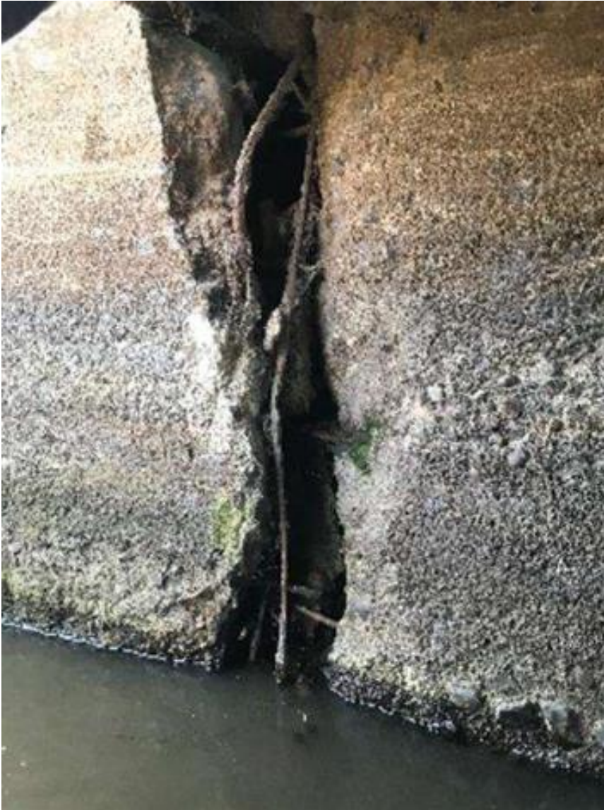
Schutte Road – Wing Wall Separation from Abutment
