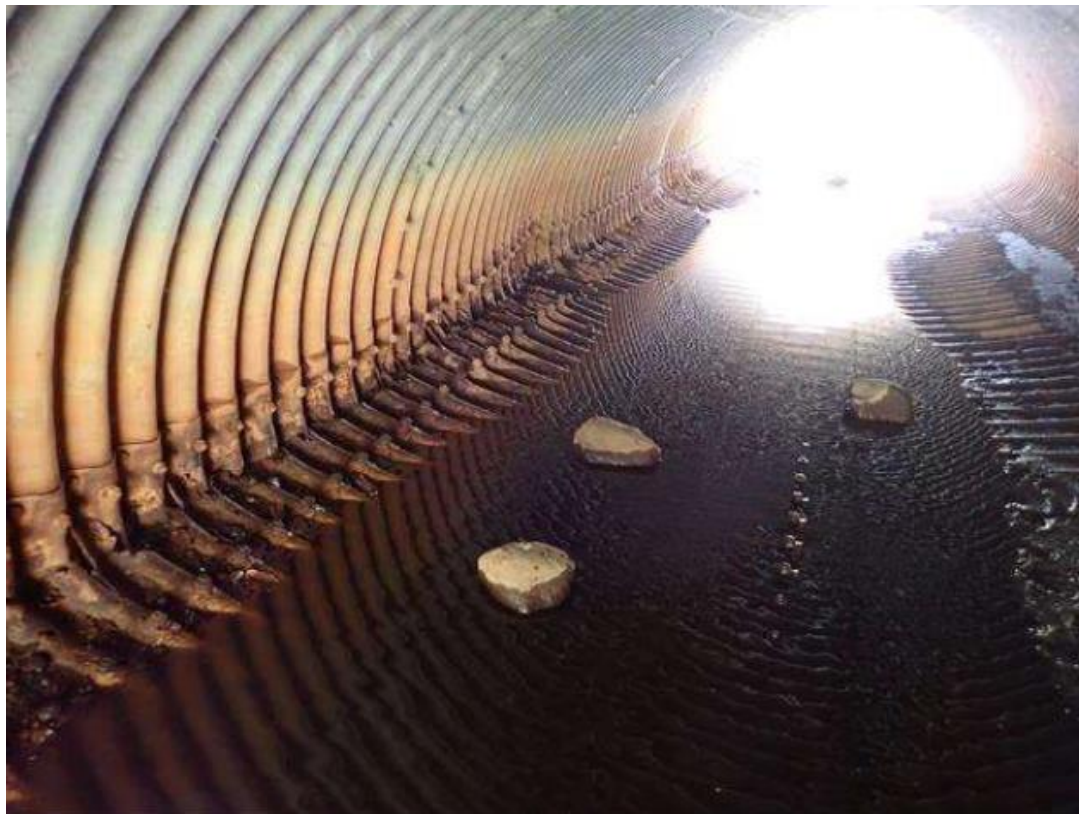
Trail Haven Road – Metal Culvert Buckling and Deterioration
