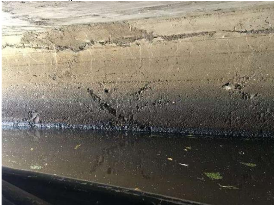
Cain Road Spalling and Cracking
