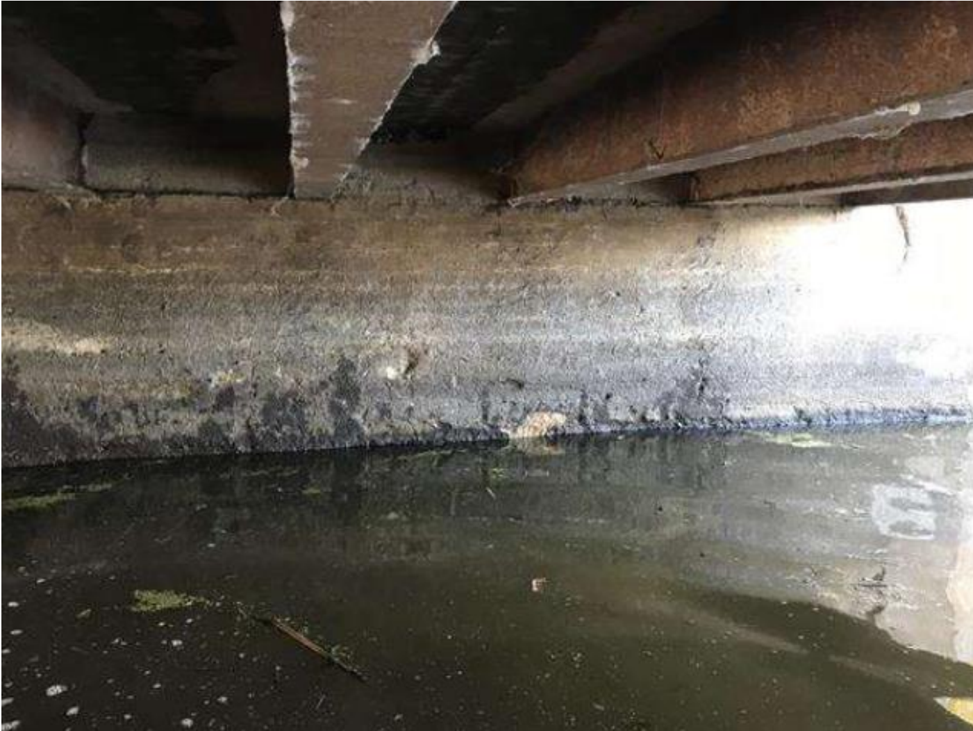
Schutte Road – Abutment and Beam Scaling and Deterioration
