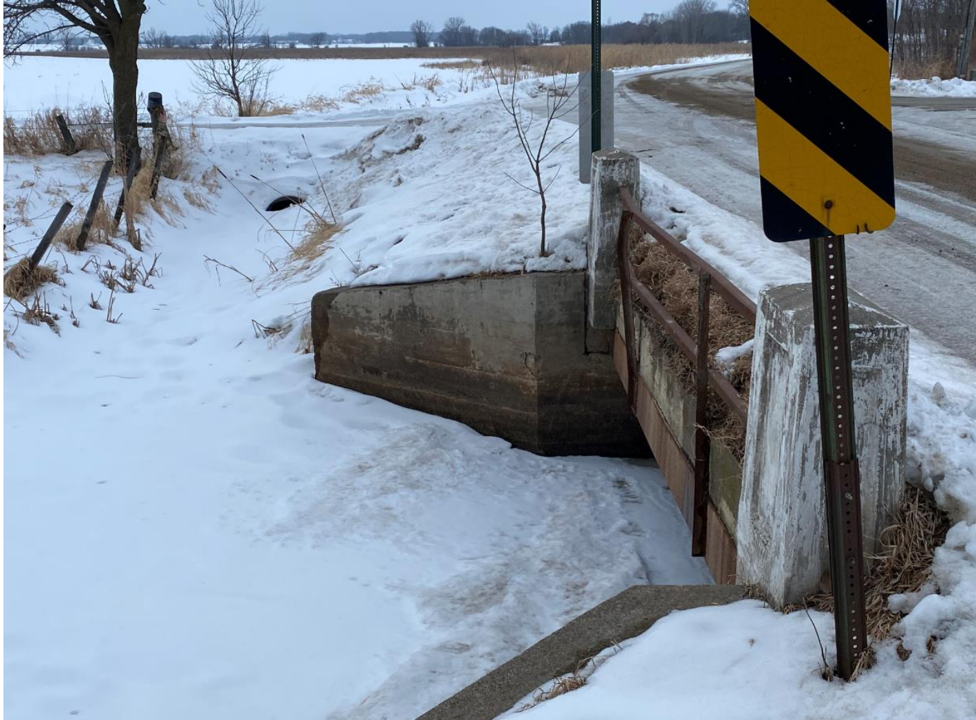
Schutte Road – Structure Aging and Deterioration
